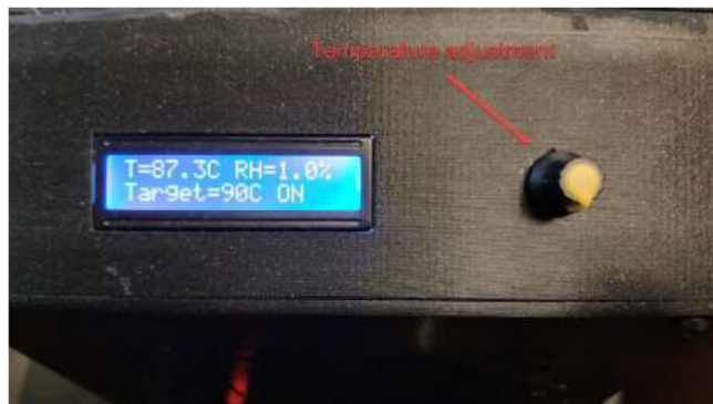
Fig. 134. Drying Chamber control panel.
