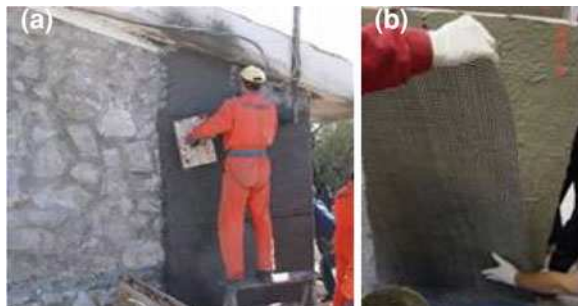
Fig. 5.10 a Practical application of TRM on masonry wall. b Strengthening of masonry specimens using TRM jackets
